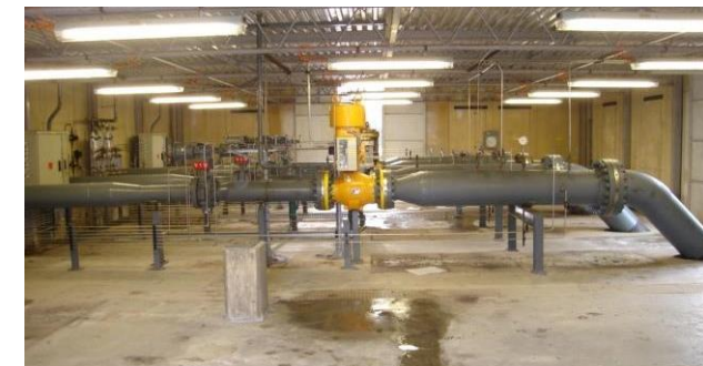
Regulators within the building
