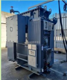
Hybrid Intelligent Transformer
