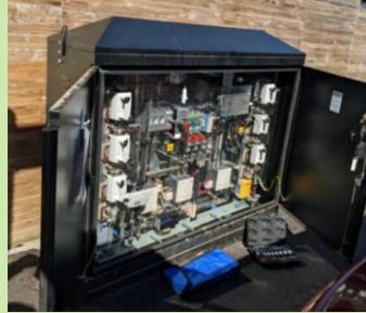
Phase Switch System
