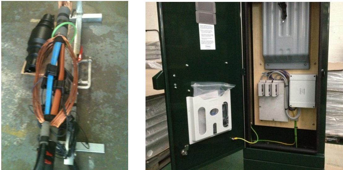
Figure 3 – Smart Joint and Marshalling Cabinet
